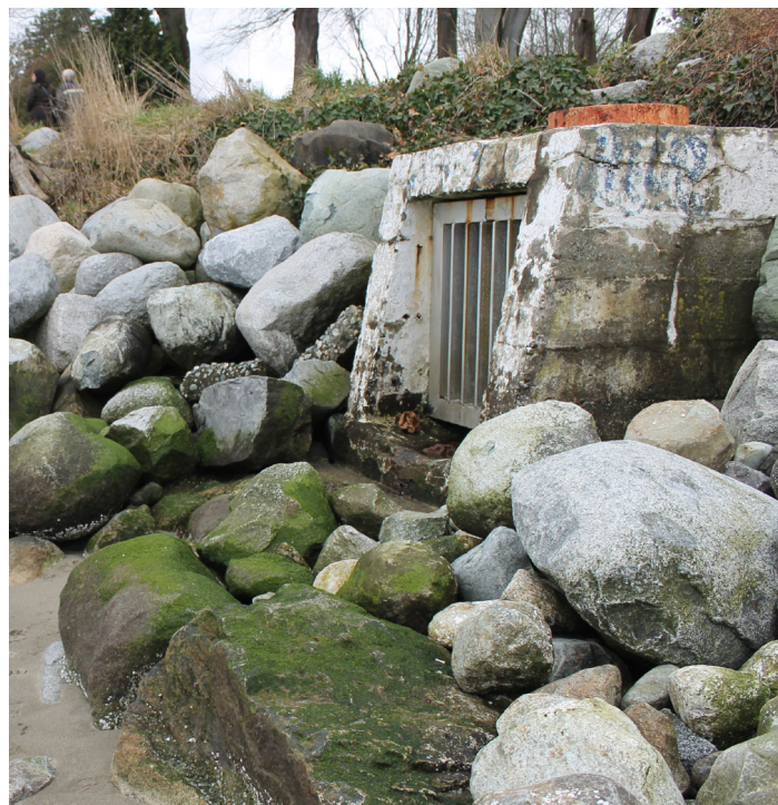
Figure 1. Combined Sewer Outfall, Comox Street, Vancouver
